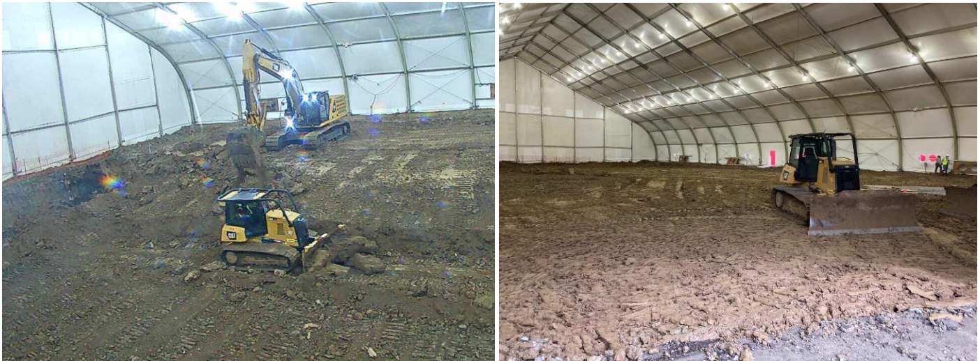
Backfilling the excavation area of the first location with clean imported soils inside of the tent.
