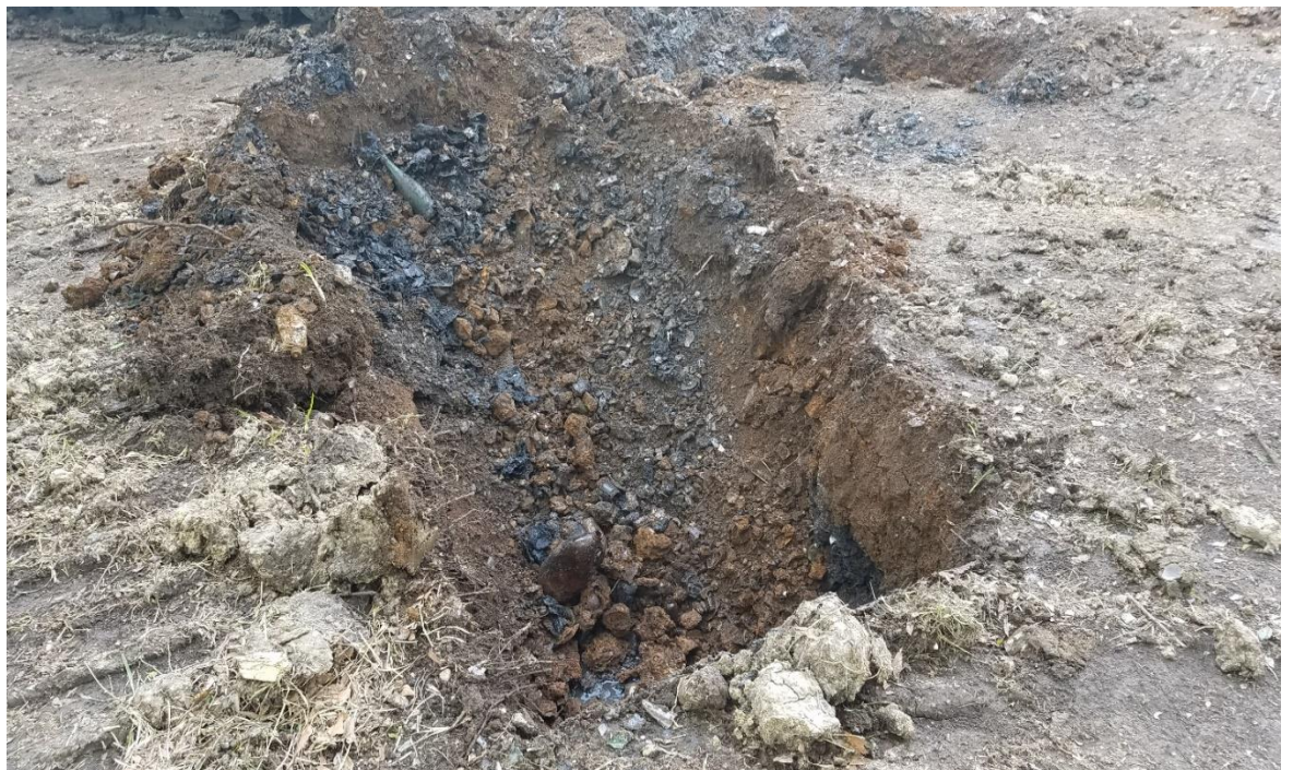
Debris from Former Gonzales Municipal Landfill Encountered East of the Tent Location
